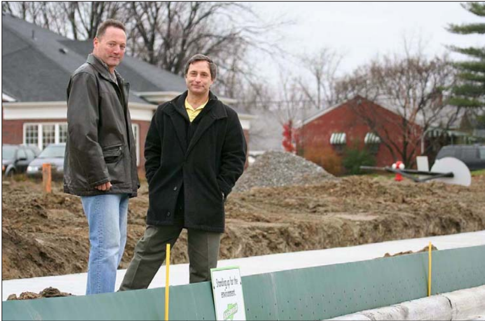
SiltShield partners Steve Mini and TDIC owner Mark D'Andreta have installed their state-of-the-art silt fencing at a project on Mound Road in Sterling Heights.
